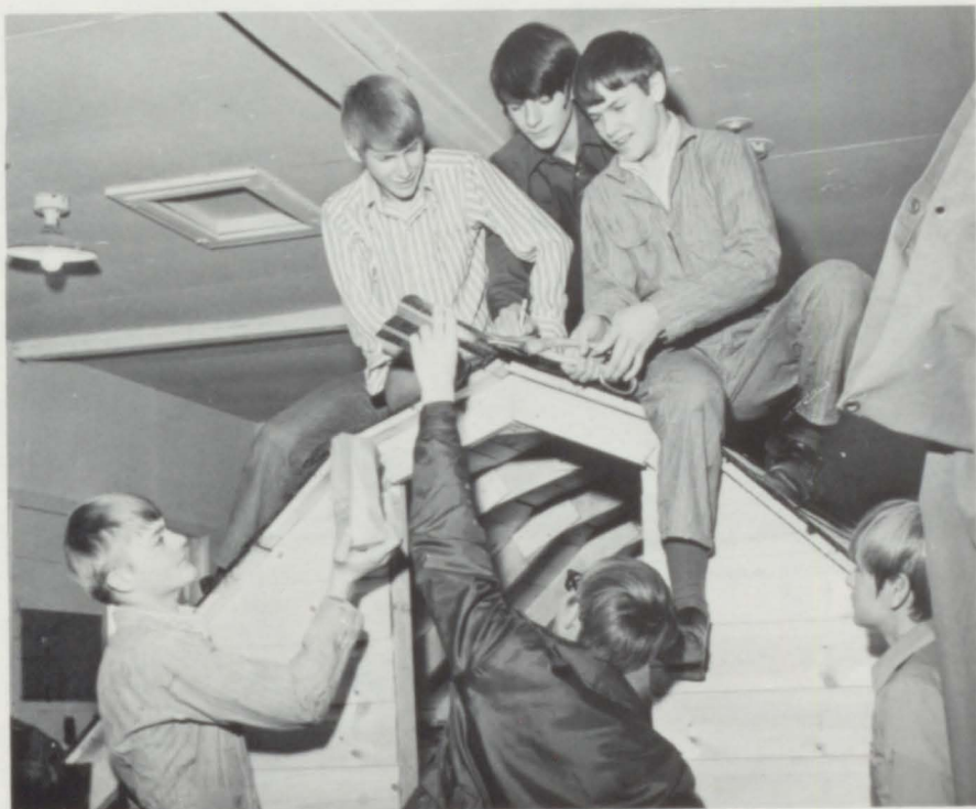
In Agriculture II, the boys enjoy shop as much as the regular classroom activities and here they are finishing a small building.
